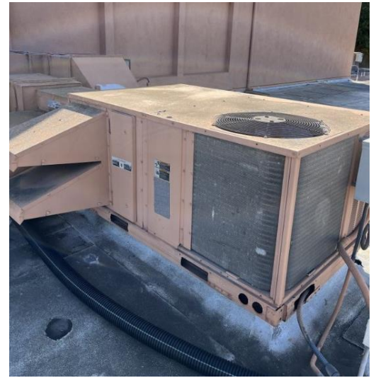
Figure 7: Rooftop Unit (RTU) with Dx Cooling + Natural Gas Heating – Ludwick Recreation Center.
