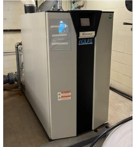
Figure 9: Natural gas boiler for pool heat at SLO Swim Center
