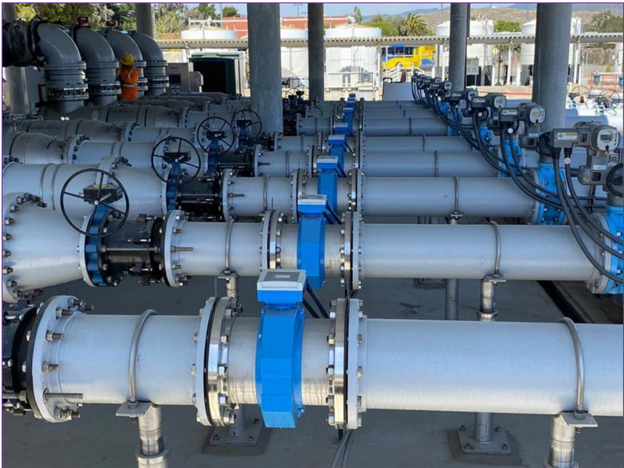
Ultraviolet Treatment at the Water Resource Recovery Facility.
