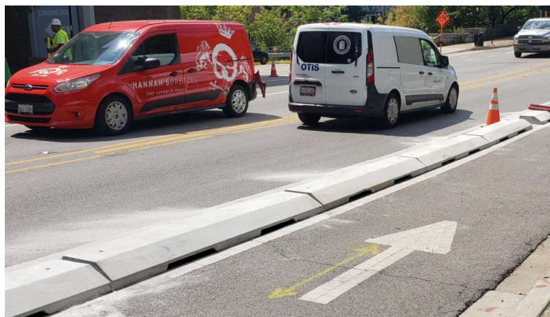
Figure 5: Example Photo of Pre-Cast Concrete Bikeway Curbs in Bid Additive Alternative for Higuera (Bridge to Margarita)
