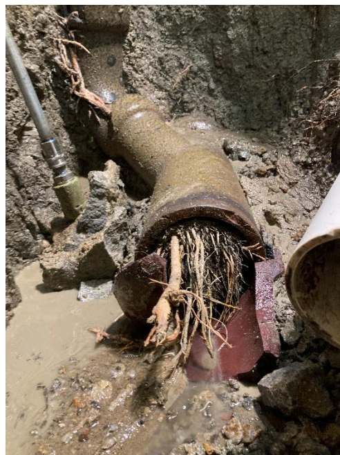
Figure 5: Private Sewer Lateral with Root Intrusion
