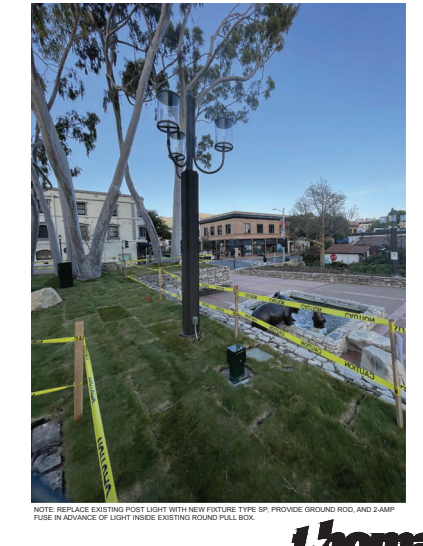
NOTE: REPLACE EXISTING POST LIGHT WITH NEW FIXTURE TYPE SP, PROVIDE GROUND ROD, AND 2-AMP FUSE IN ADVANCE OF LIGHT INSIDE EXISTING ROUND PULL BOX.
