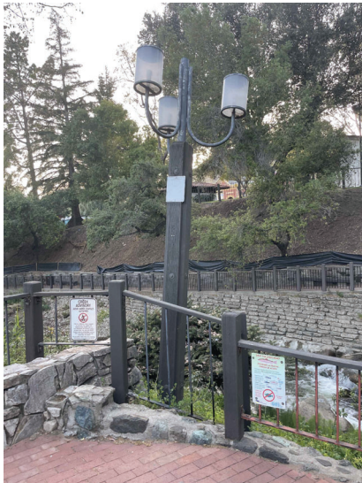
NOTE: REPLACE EXISTING POST LIGHT WITH NEW FIXTURE TYPE SP, PROVIDE NEW PULL BOX, GROUND ROD, AND 2-AMP FUSE IN ADVANCE OF LIGHT INSIDE NEW PULL BOX.
