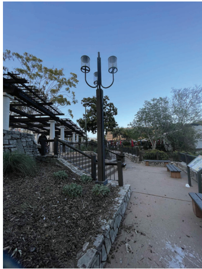
NOTE: REPLACE EXISTING POST LIGHT WITH NEW FIXTURE TYPE SP, PROVIDE NEW PULL BOX, GROUND ROD, AND 2-AMP FUSE IN ADVANCE OF LIGHT INSIDE NEW PULL BOX.
