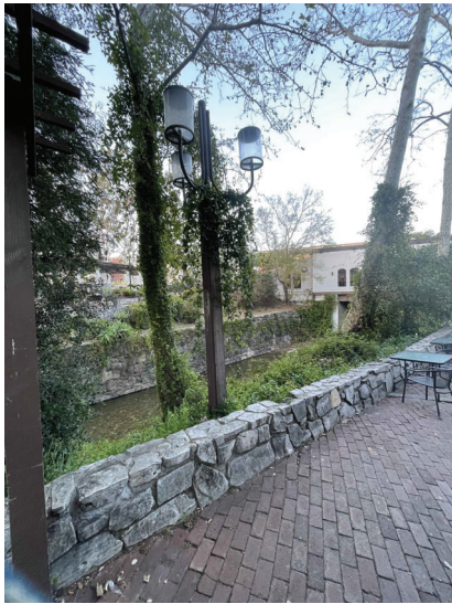
NOTE: REPLACE EXISTING POST LIGHT WITH NEW FIXTURE TYPE SP, PROVIDE NEW PULL BOX, GROUND ROD, AND 2-AMP FUSE IN ADVANCE OF LIGHT INSIDE NEW PULL BOX.
