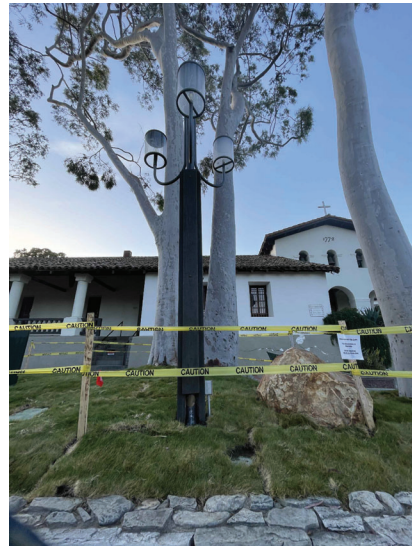
NOTE: REPLACE EXISTING POST LIGHT WITH NEW FIXTURE TYPE SP, PROVIDE GROUND ROD, AND 2-AMP FUSE IN ADVANCE OF LIGHT INSIDE EXISTING ROUND PULL BOX.
