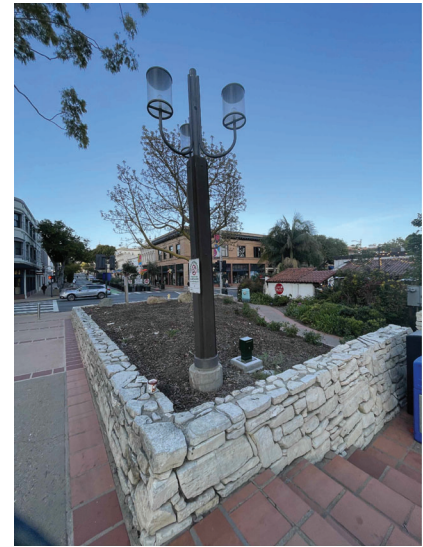
NOTE: REPLACE EXISTING POST LIGHT WITH NEW FIXTURE TYPE SP, PROVIDE GROUND ROD, AND 2-AMP FUSE IN ADVANCE OF LIGHT INSIDE EXISTING ROUND PULL BOX.
