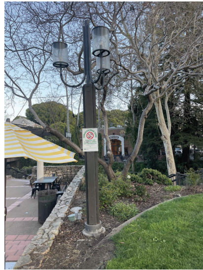
NOTE: REPLACE EXISTING POST LIGHT WITH NEW FIXTURE TYPE SP, PROVIDE GROUND ROD, AND 2-AMP FUSE IN ADVANCE OF LIGHT INSIDE EXISTING ROUND PULL BOX.
