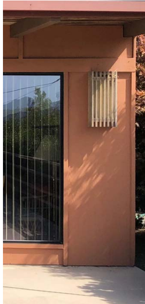
Page-Selkirk House: Plywood sheathing, battens, fixed glass, V-groove shiplap soffit, plain beams, wood-strip lamp
