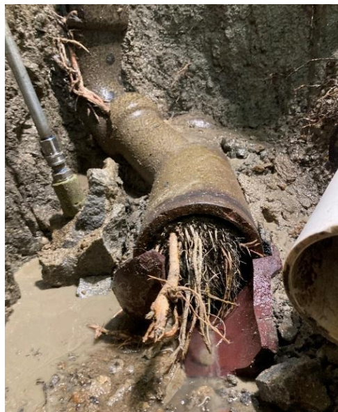
Figure 3: Private Sewer Lateral Root Intrusion
